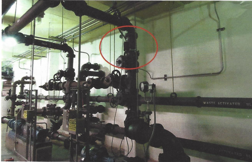
One water conditioning unit treated flows just after the discharge of the thickened waste activated sludge pump, which is about 23 m (75 ft) upstream of the centrifuge. Chuck Glessner
