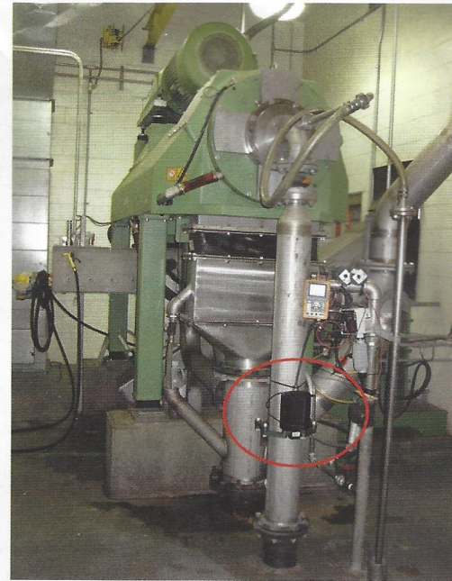
HydroFLOW staff installed a pair of water conditioning units. The one pictured about 1.5 m (5 ft) upstream of the solids entrance to the facility's centrifuge. Douglas Lee Miller
