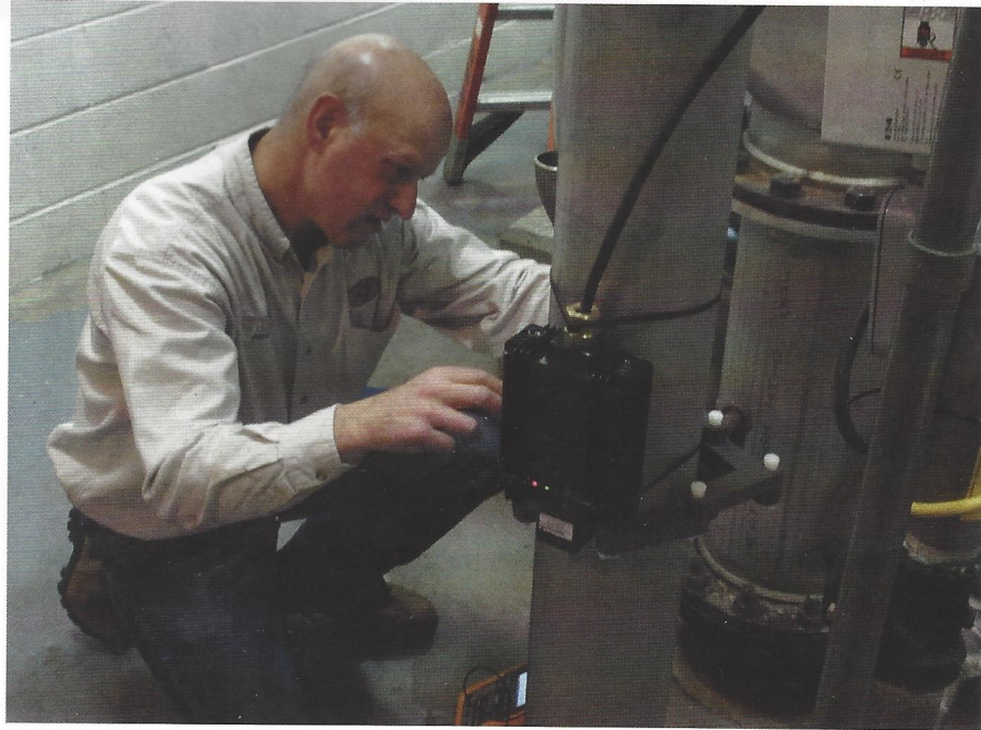
Douglas Miller installs a water conditioning unit on the centrifuge feed piping. Chuck Glessner
